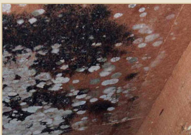
Fig. 3. Mould in the building structure
